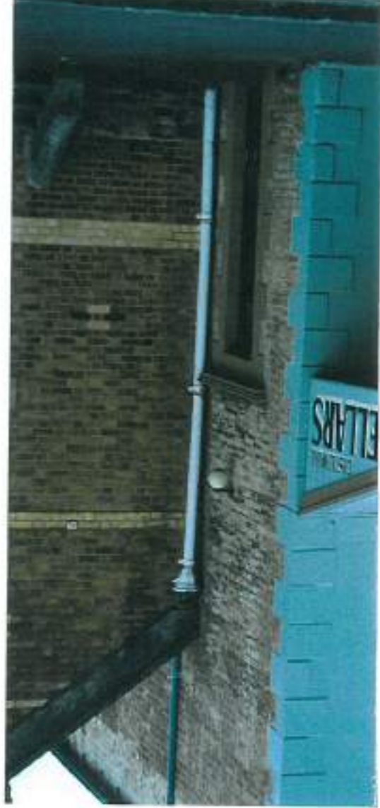
top left: A small lamp left on at night would add to the charm, interest and safety of this space. top and bottom right: The stone lined drains are a priceless, cohesive streetscape element and need to be conserved. bottom left: Well lit shops add much to the town's night time appeal.
