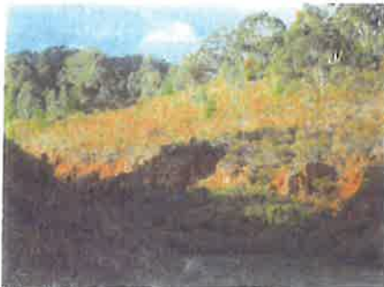
Eroded creek bank along Fryers Road With regrowth of Box- Ironbark forest
