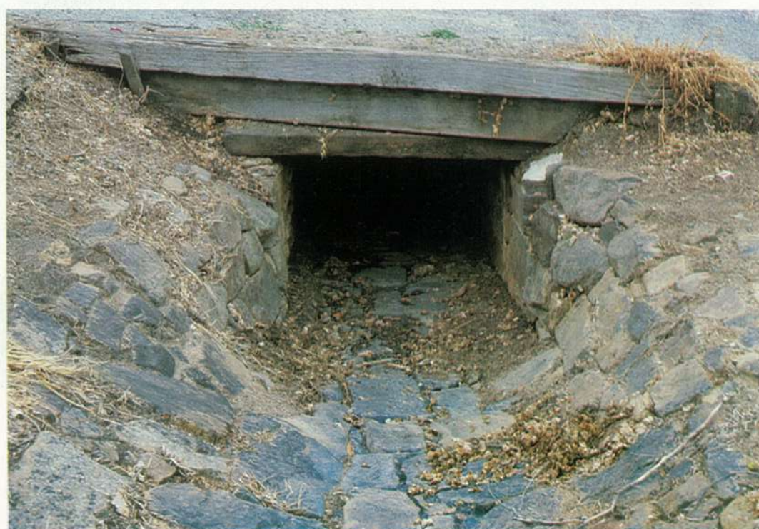
Storm water channel, of local stone, dating back to the mid-nineteenth century.
