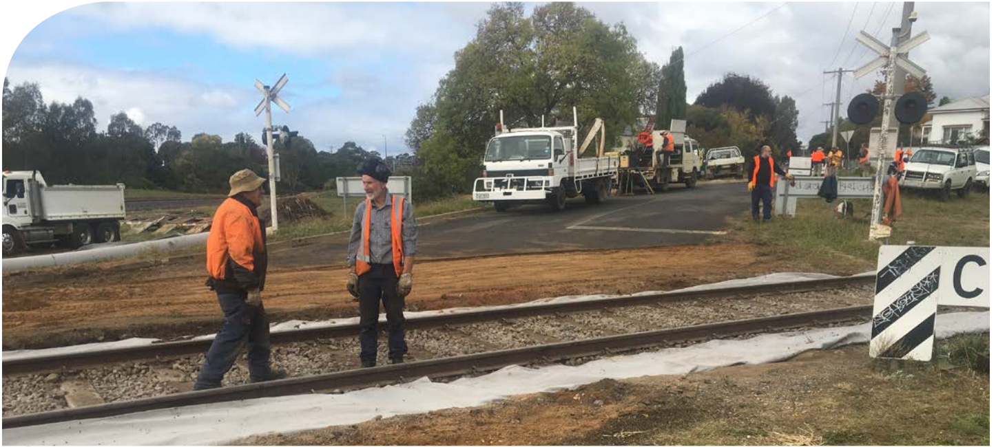
Replacing the old timber railway sleepers on a railway level crossing in Rowe Street, Castlemaine
