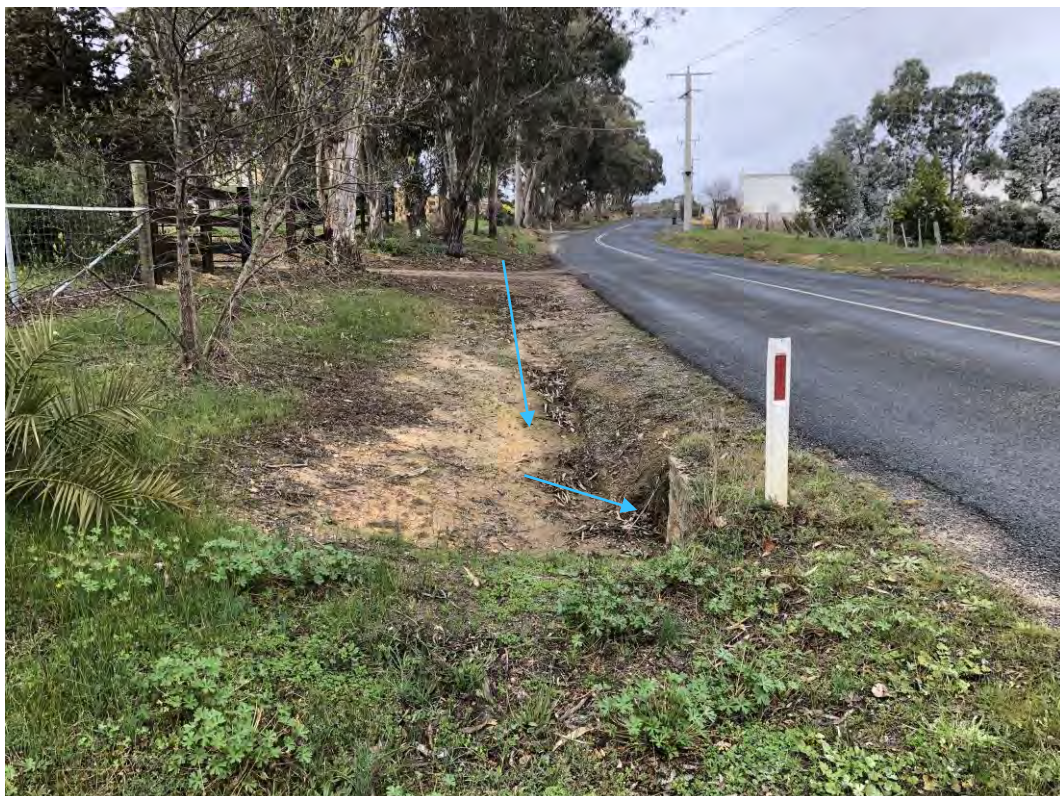
Photo 6 – View S along Blakeley Road, culvert on roadside drain, flowing to site
