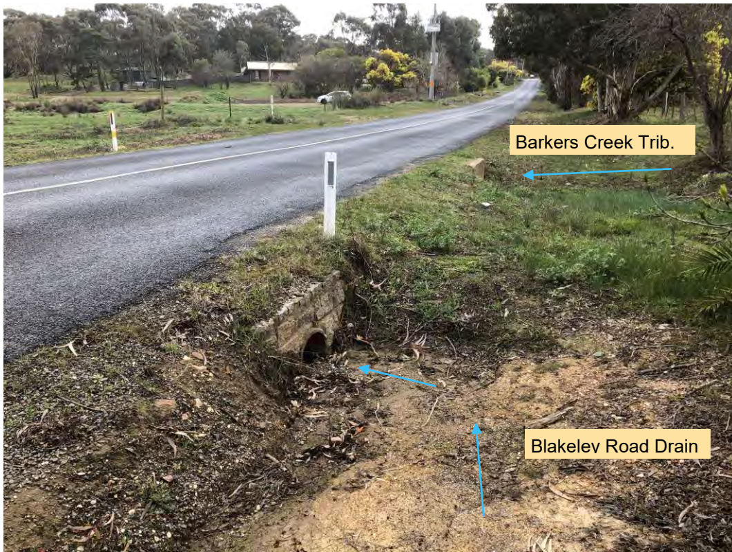
Photo 5 – View N along Blakeley Road, 2 sets of culverts flowing west under road
