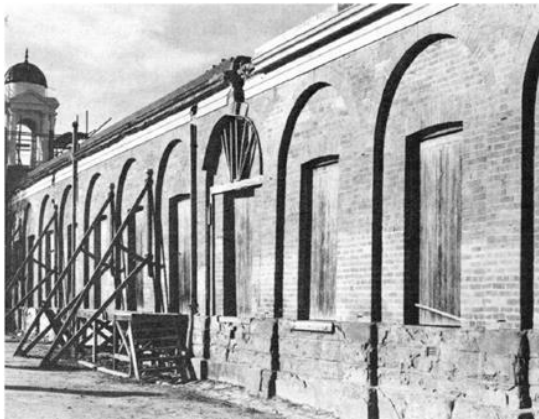
Figure 181: Structural remediation works, Castlemaine Market, June 1969 (Source: National Trust, Castlemaine and the Market , p.5)
