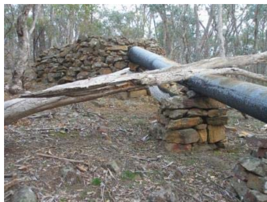
Figure 26: Collapsed siphon and support structure at Devils Gully.
