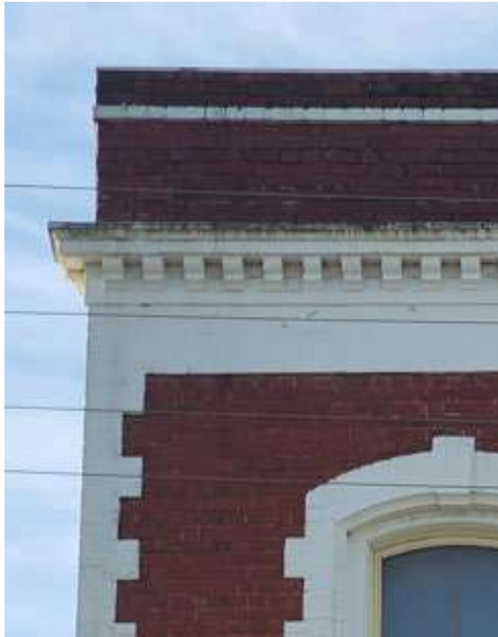
Figure 8. The upper-level façade retains contrasted detailing, all originally finished in face brick (now overpainted). (Source: GML 2021)
