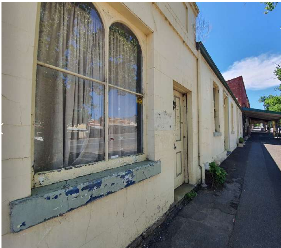
Figure 8. 1877 addition finished with ruled render (now overpainted) and decorative four-pane window. Note the ruled render has been applied across the entire street frontage. (Source: GML 2021)
