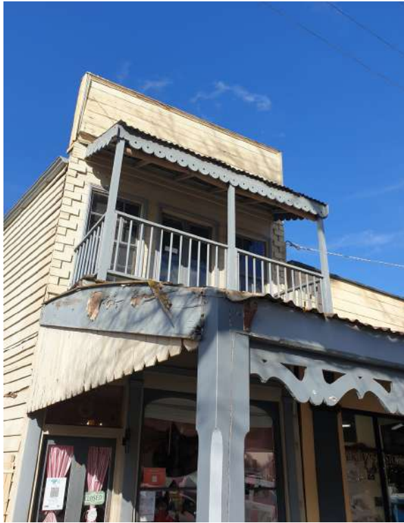
Figure 11. The upper-level façade retains flat parapet, timber quoining to the edges, verandah with scalloped detailing, timber verandah posts and balustrades, and timber-framed sash windows. Note the timber valance and posts on the ground level is not original. (Source: GML 2021)
